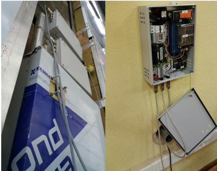
Figure 4: (left) 2 devices installed inside the ventilated façade and (right) one device indoors, showing the internal elements.
